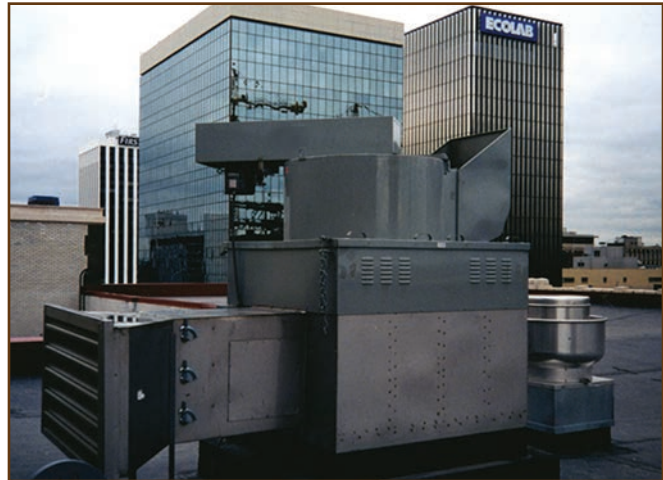
Photo 2: High velocity, vertical discharge, centrifugal roof fan with a dilution air intake.
